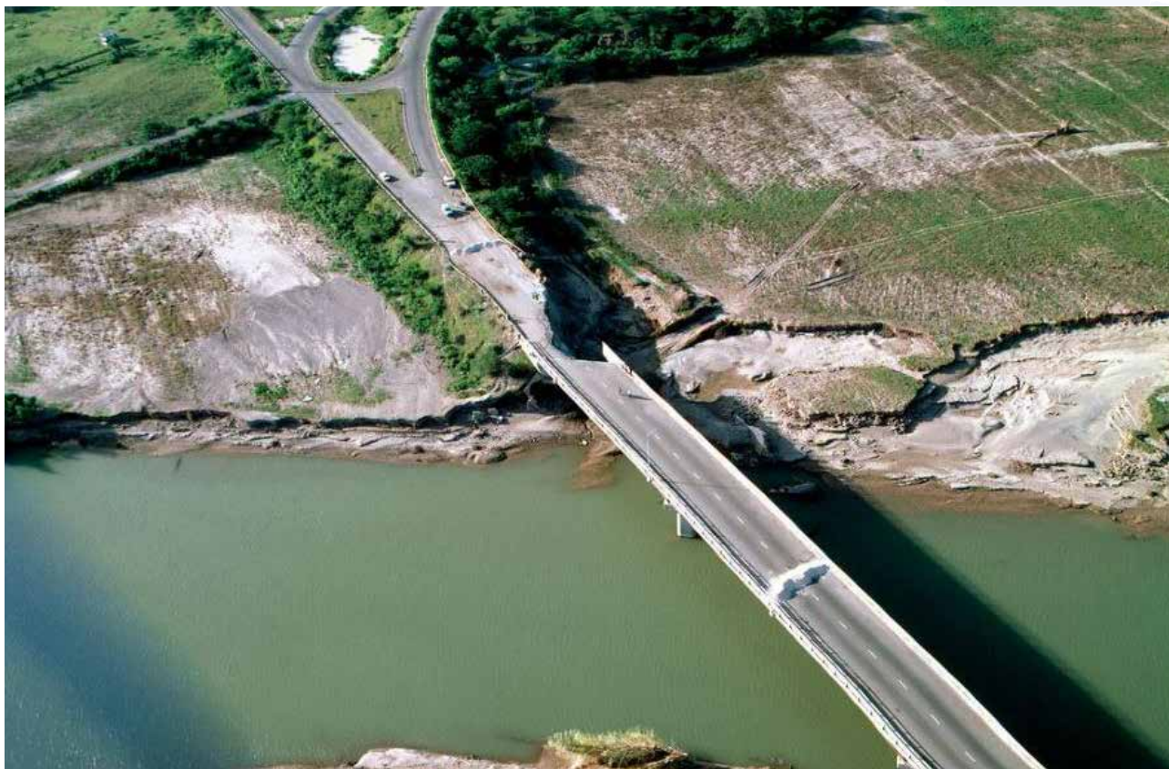
This bridge in May Pen Jamaica was damaged by flooding. Photo ©United Nations/M.Grant.
