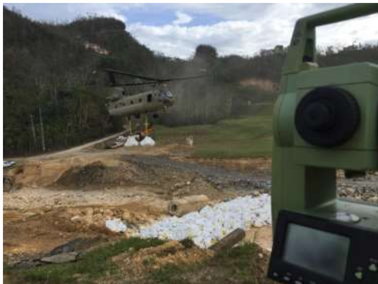
Figure 7. US Army Corps of Engineers' personnel collaborating in the mitigation efforts at Guajataca Dam after hurricane Maria. (Seda, 2017)
