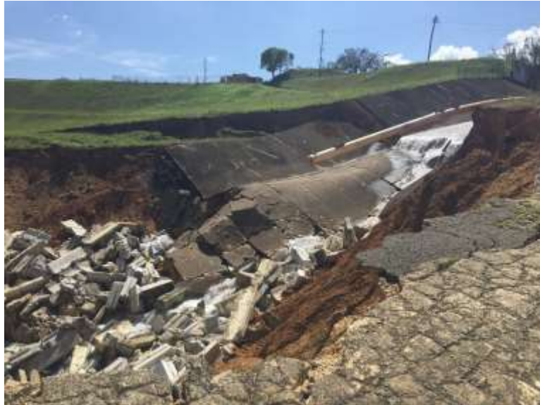
Figure 4. Erosion at base of dam. (Seda, 2017)
