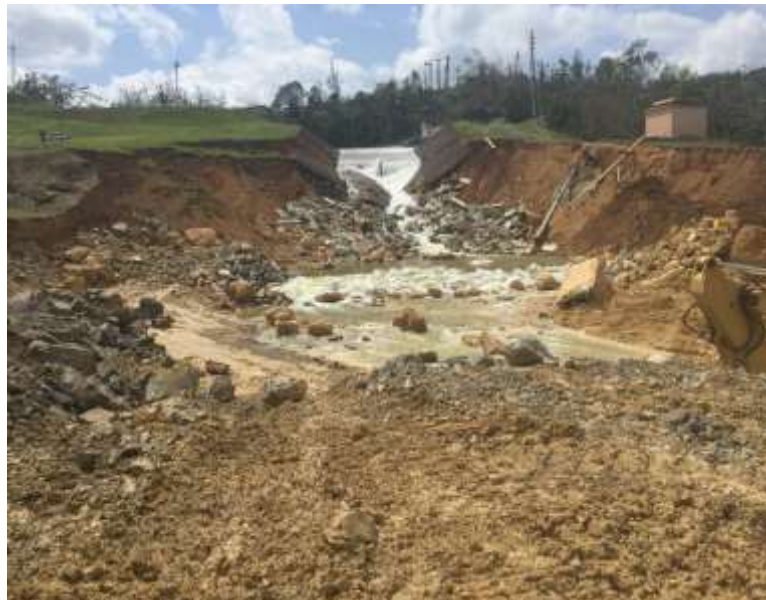
Figure 5. Erosion at base of dam. (Seda, 2017)
