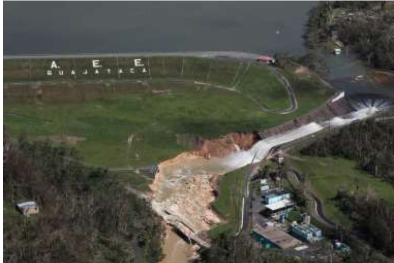
Figure 6. Aerial view showing the damage to the Guajataca Dam in the aftermath of Hurricane Maria. (Alvin Baez/ Reuters, 2017)
