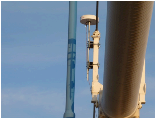
Figure 5. GNSS light weight choke ring antenna located on the suspension cable at location C.
