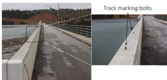
Figure 3: Two of the permanent geodetic bolts installed on the crest that serve as target points for geodetic deformation monitoring.
