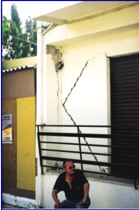
1 a . Disconnection of an infill brickwall from the load bearing system.
