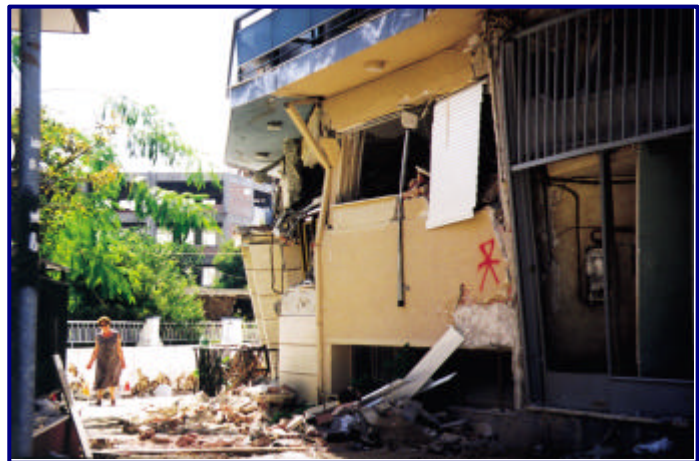
3. Fracture of a beam at the perimeter of the load bearing system, close to its corner
