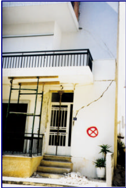
5 b . Cracking of shear wall at the corner of the building
