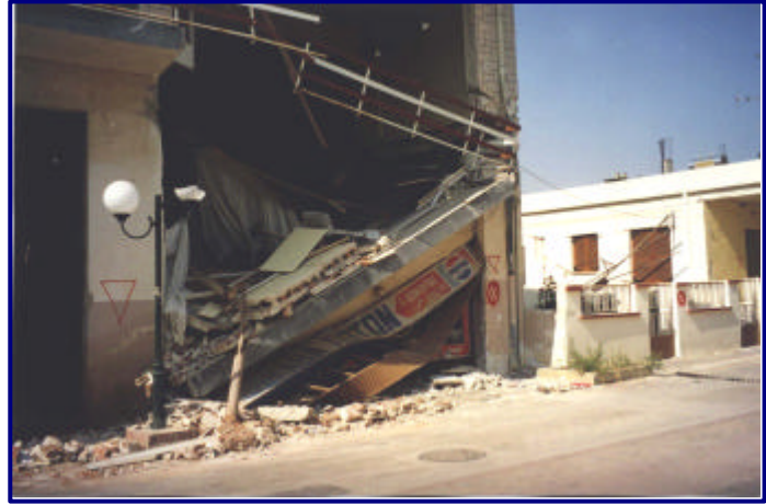
2. Collapse of a reinforced concrete slab due to yielding of a reinforced concrete column
