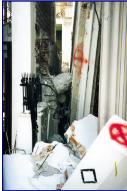
5 c . Inclination of a shear wall due to lack of stiffness in the perpendicular direction to its surface
