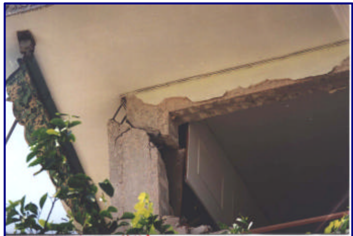
4. Disorganization of a beam to column joint
