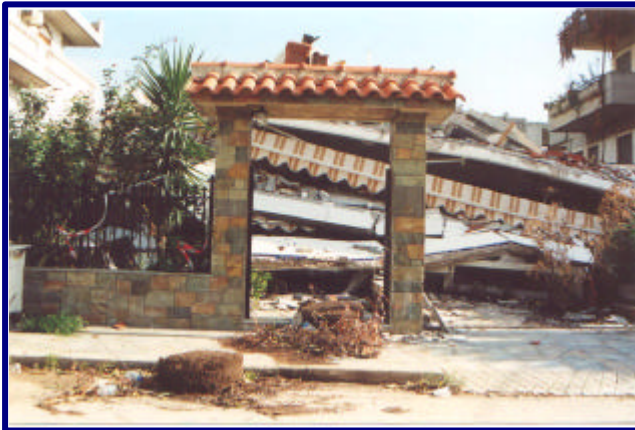
7 a . Collapse due to total failure of columns
