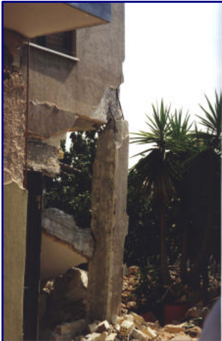
5 a . Overloading of a corner column due to seismic action. The lack of adequate stirrups is evident.
