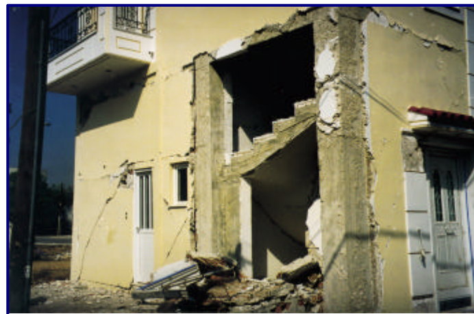
8. Absorption of seismic energy at the region where there is concentration of large mass of reinforced concrete
